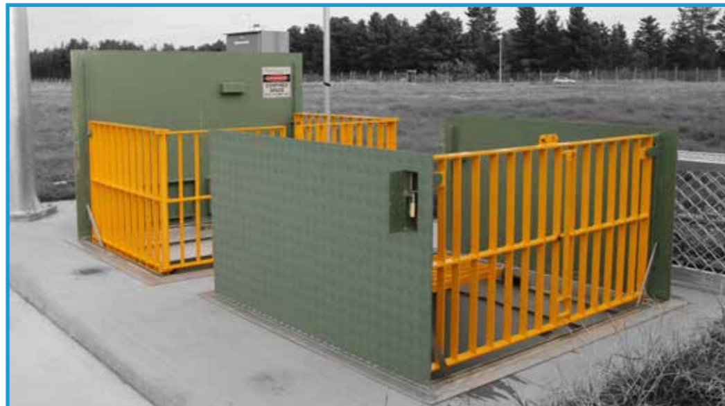
Project 15638 | Safety Access Cover for Pump Station
